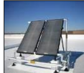
Solar Water Heating
